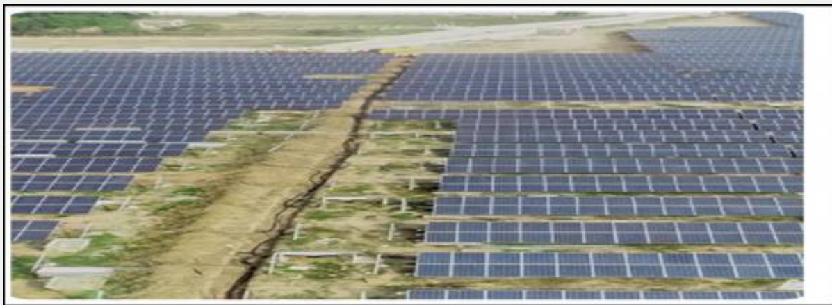
Solar Park (30 MW) at Manuguru, SCCL
