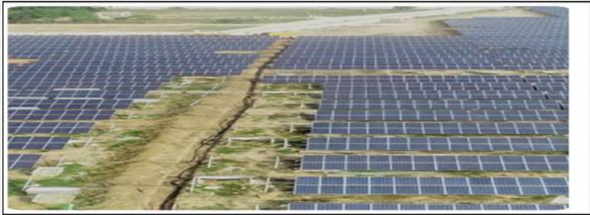
Solar Park (30 MW) at Manuguru, SCCL
